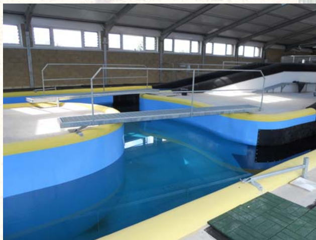
Week 30: Rubber padding fitted, walkways and bridges complete, painting dry and water rising!
